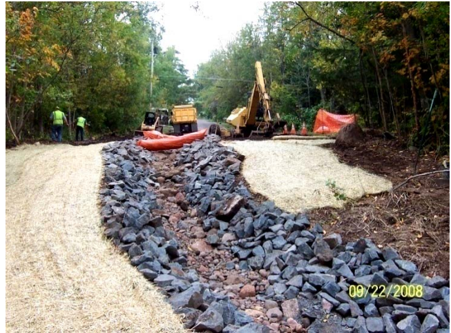
This rock chute cleans and cools down runoff before it enters Miller Creek at 22 nd Ave. W.
