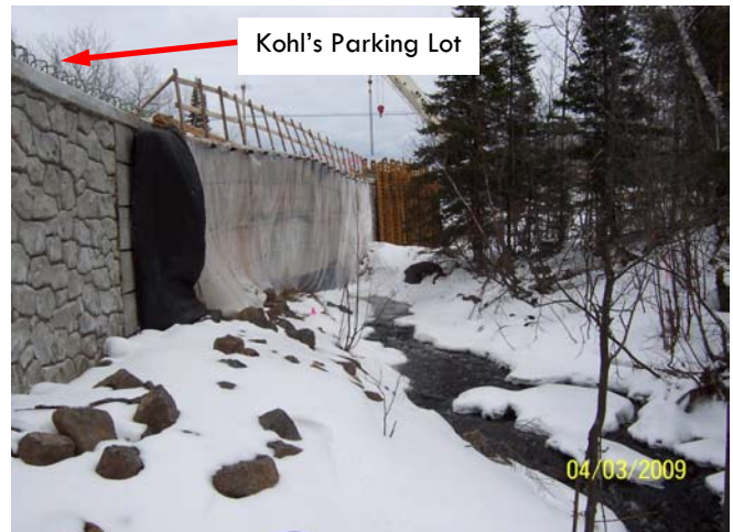
A new retaining wall was constructed along Miller Creek below the Kohl's parking lot during construction near the Mall.
