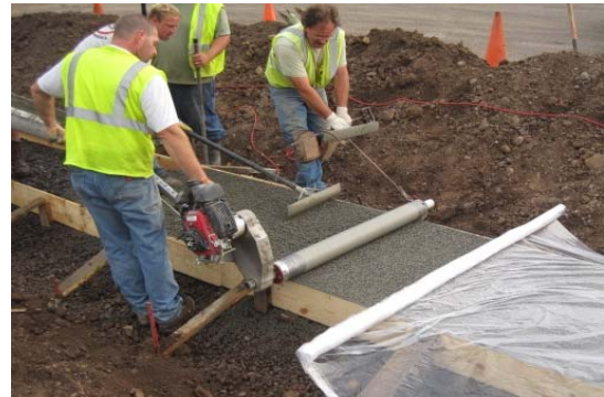
The pour shows the special concrete mix being laid in the trough; water which doesn't infiltrate directly down is carried through drain pipes to the rain garden.
